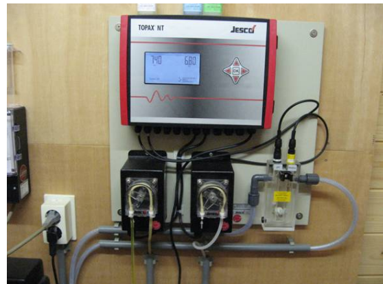
Redox sensor to measure the level of TwinOxide®
